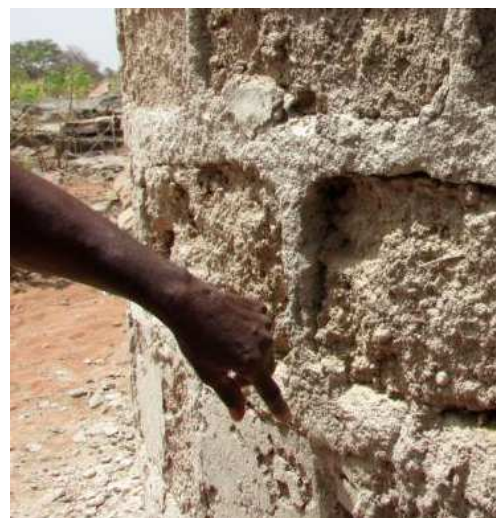
Crumbling, leaking water tank in need of repair.
